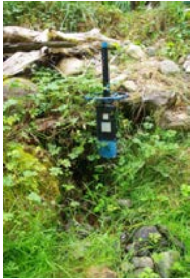
Photograph 1: Millard Creek side channel inlet control valve – 22 nd of August 2012
